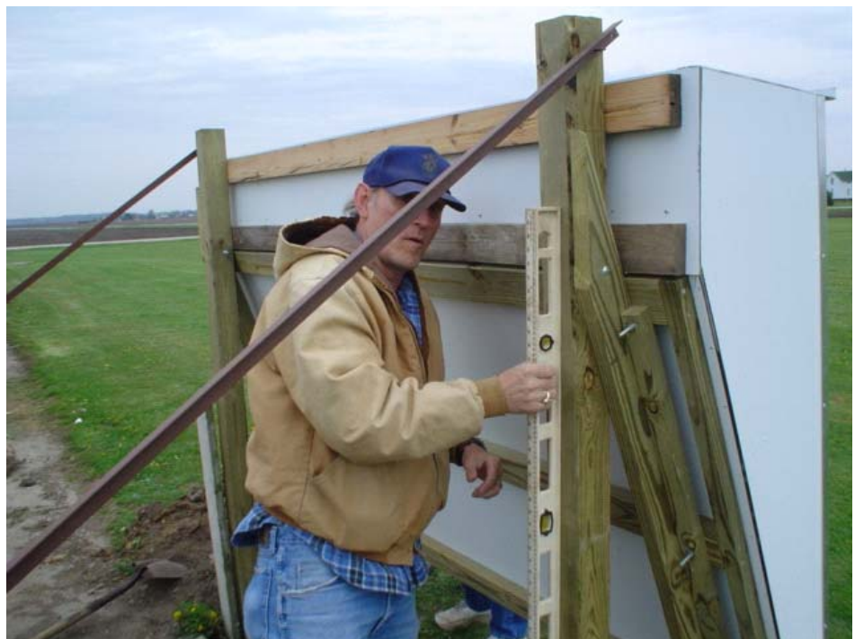
Denny Wallen works on new frequency board at the field cleanup day on April 24th.
